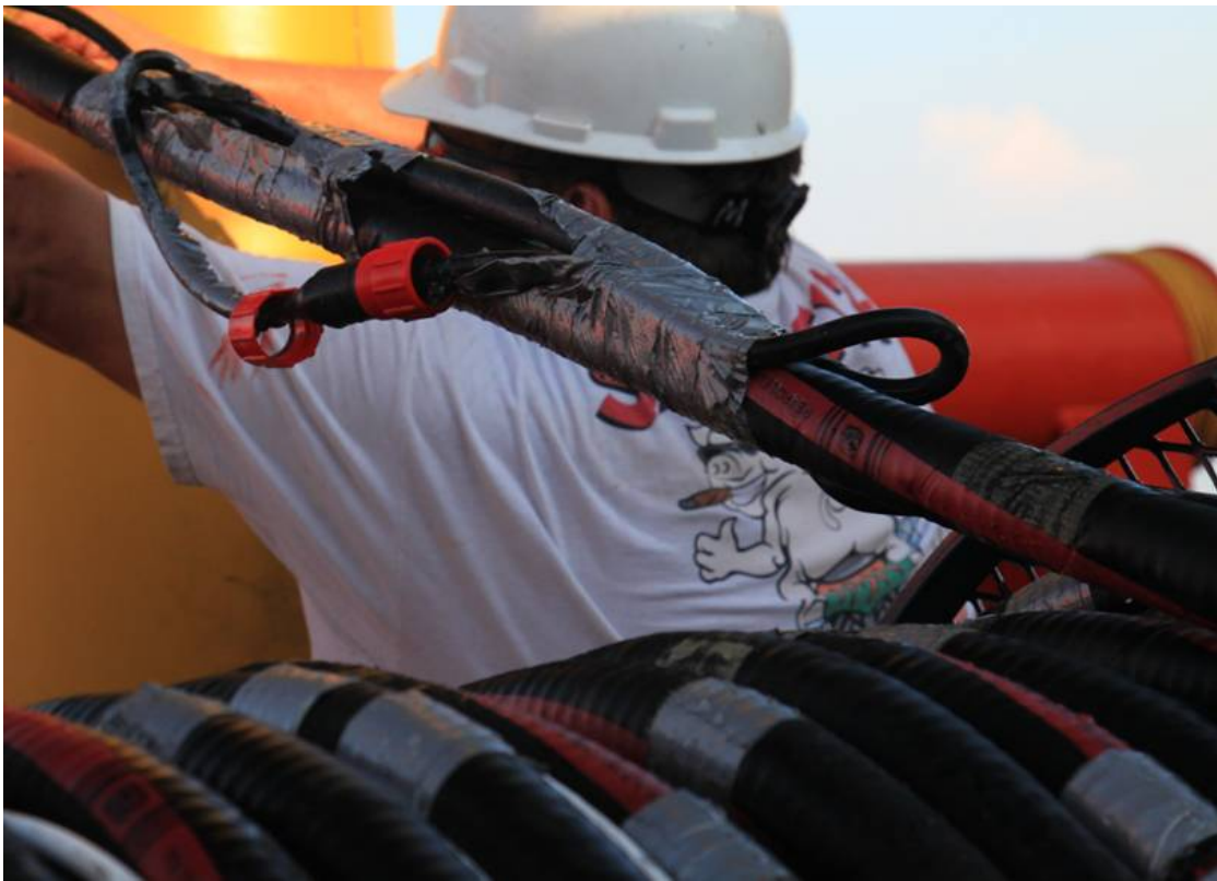
Photo 6. Example of underwater electrical connectors that pull apart when under tension.
