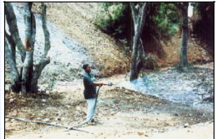
Figure 3.8. Hydroseeding side slopes and outside rim of a sediment basin (Estate New Herrhut, St. Thomas, 1998).
