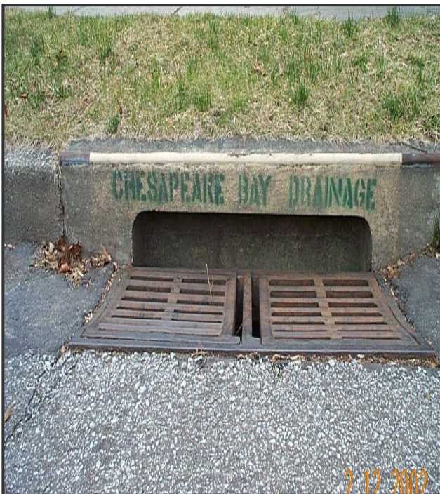
Gutter Accumulation Rating of 1
