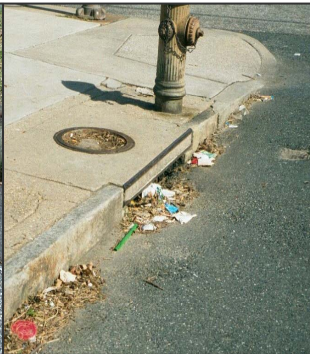
Gutter Accumulation Rating of 3
