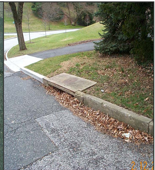
Gutter Accumulation Rating of 5
