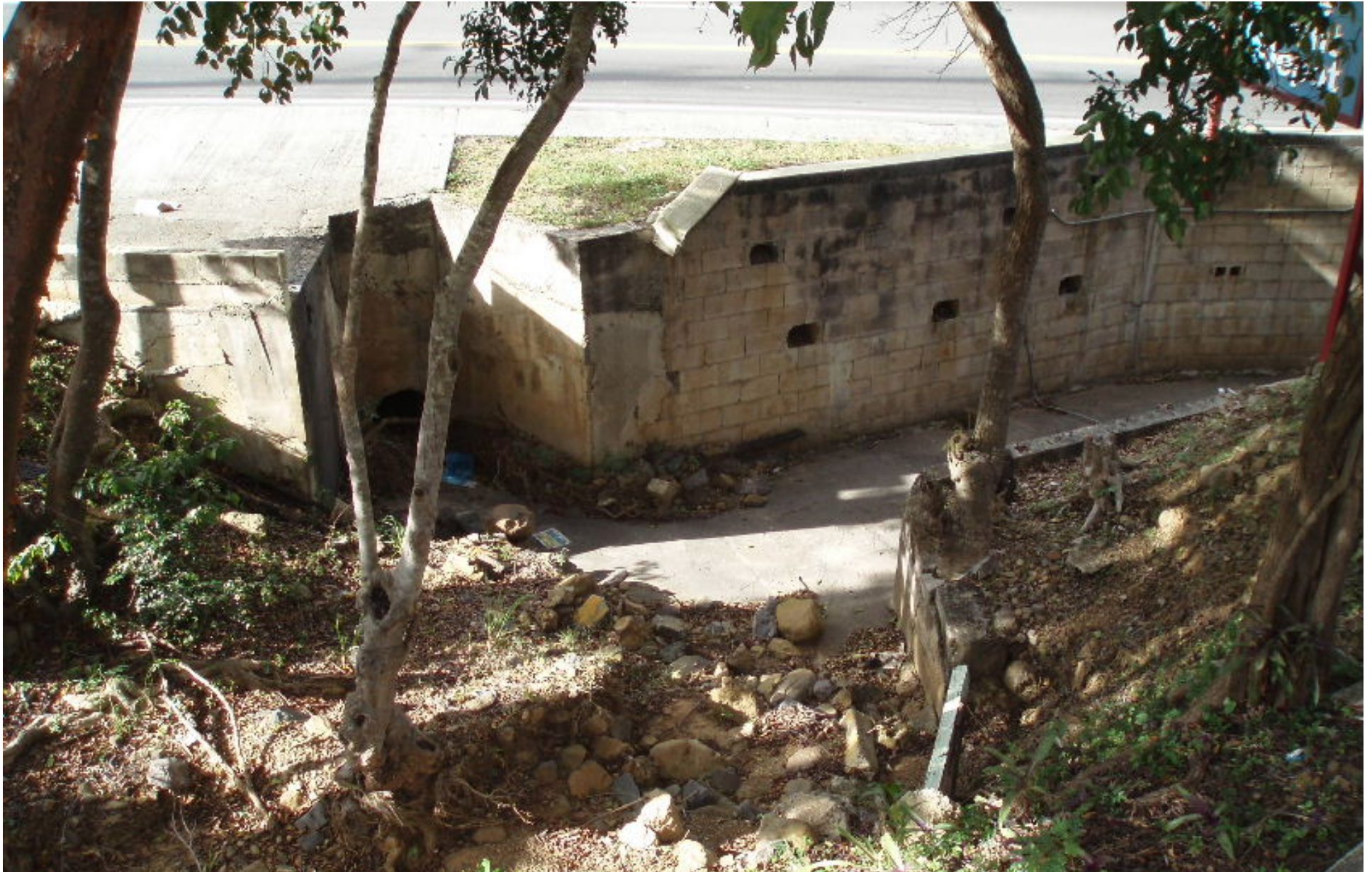
Guts encroached by roadways, piped, and used for dumping
