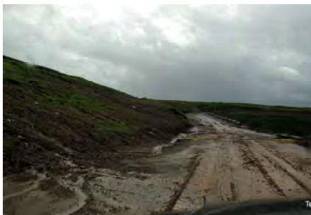
Road to landfill subject to erosion and washout during heavy rainfall.
