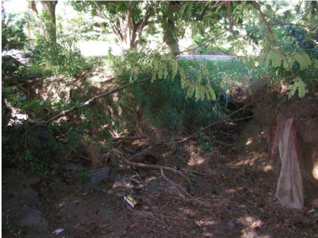
Figure 8.7. West gut erosion and trash.
