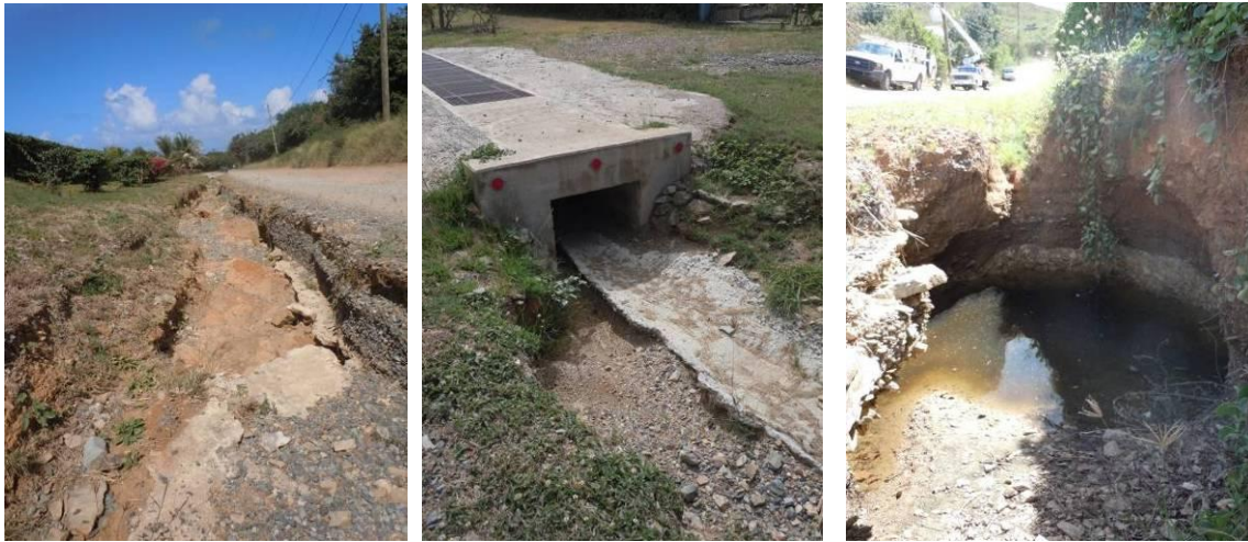
Figure 4.5. Erosion gullies are undermining the unpaved Seven Flags Rd. (left), scouring around and under existing infrastructure (middle), and creating dangerous public hazards (right).
