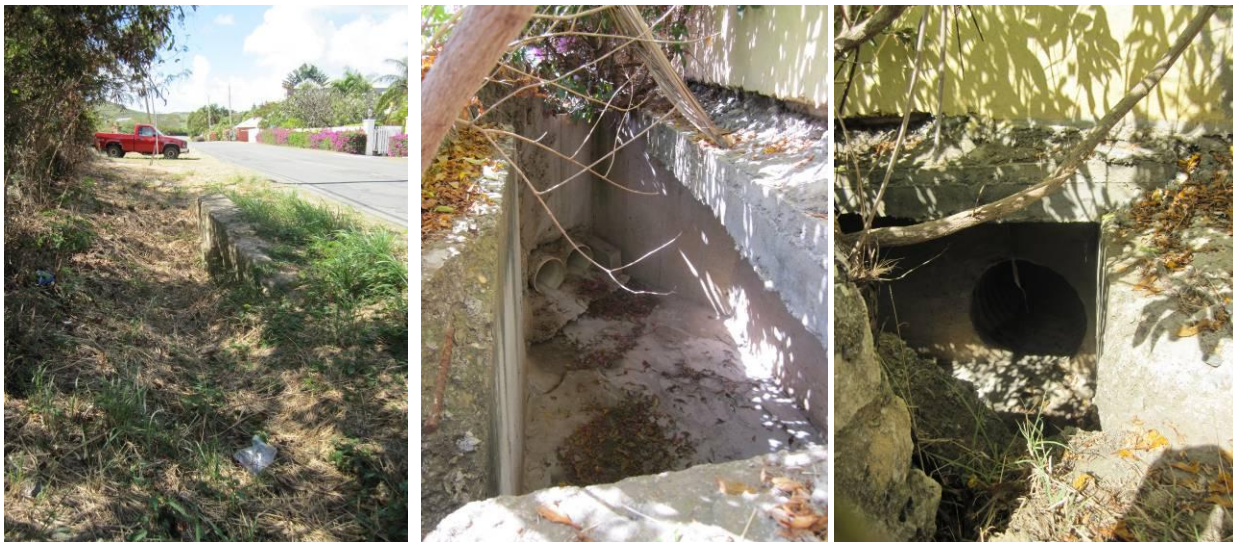
Figure 4.36. Upstream end of 24-inch culvert and headwall; Sierra Verde Rd. in the background (left); the two PVC pipes in the drainage structure at the downstream end of the culvert (middle); and the ultimate discharge pipe to the bay where runoff leaves the drainage structure (right).
