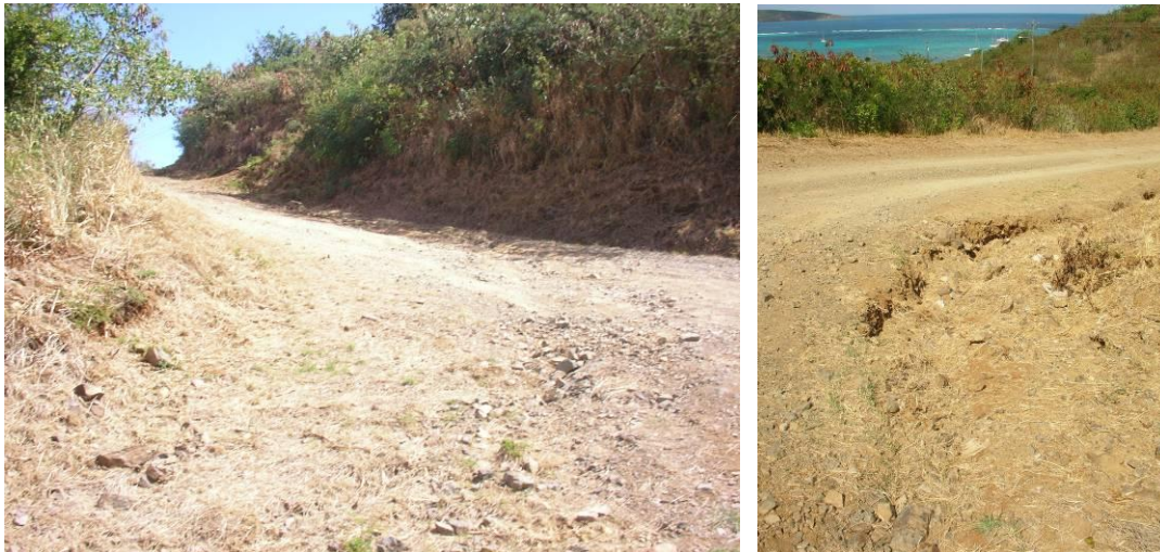
Figure 5.7. Gullying and erosion observed along Ridge Rd.
