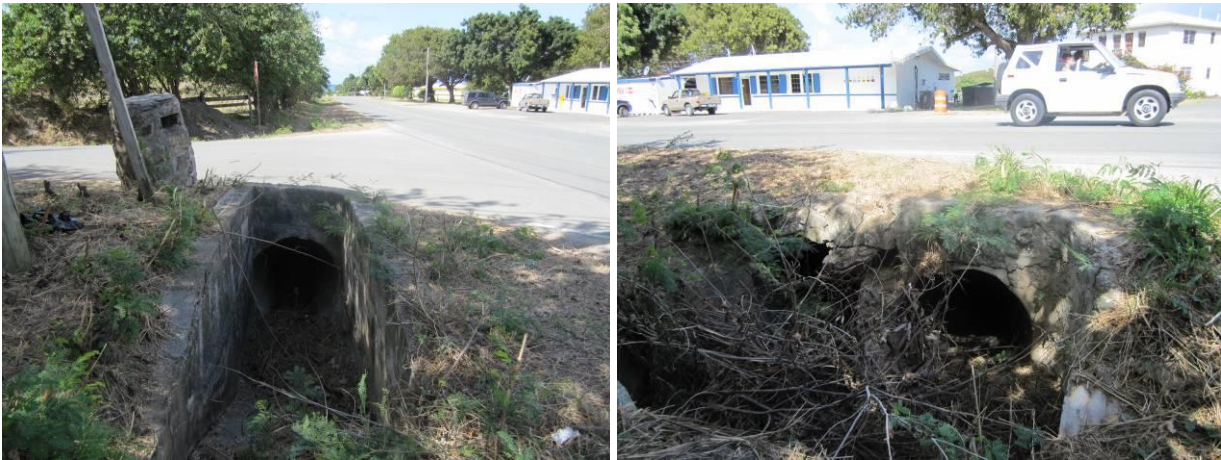
Figure 4.14. 30-inch culvert under Solitude Rd (left) and two 30-inch culverts under East End Rd., leading to a 48-inch culvert that discharges to Coakley Bay (right).
