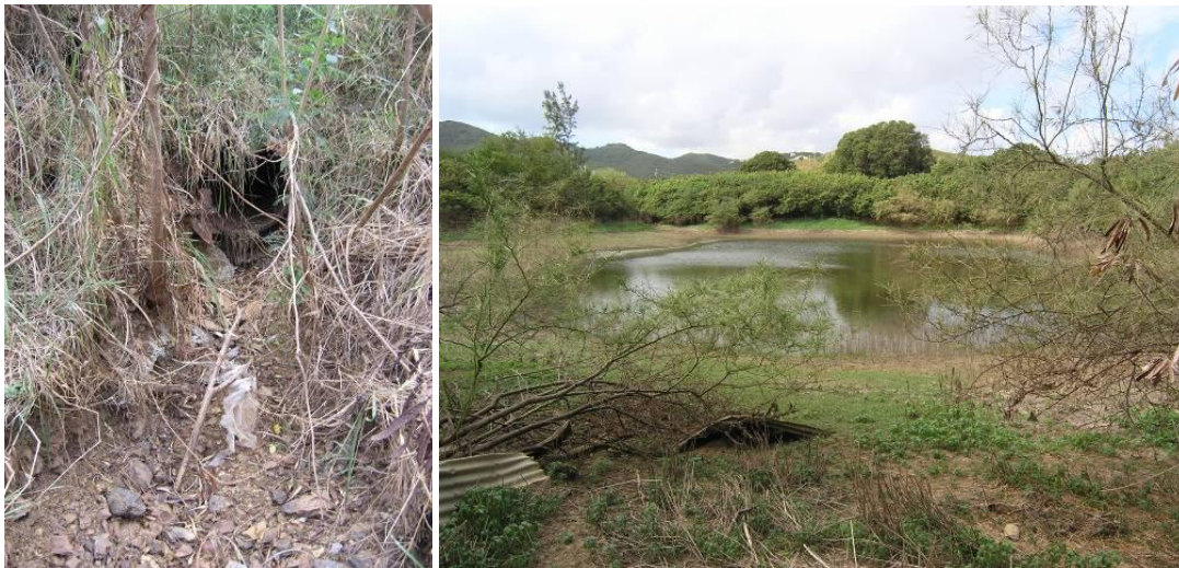
Figure 4.27. Scouring was observed downstream of this culvert (left), which leads to sedimentation of the large pond downstream (right).
