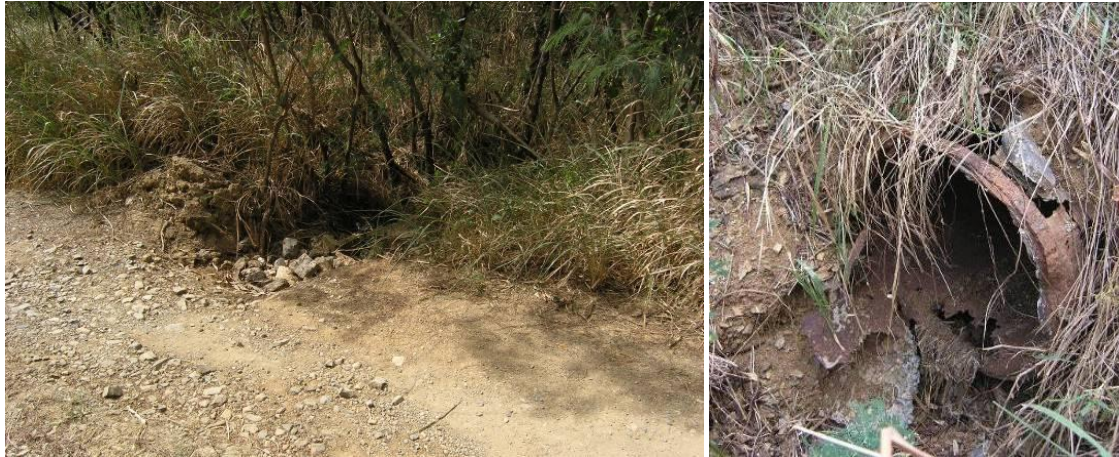
Figure 4.26. The upstream end of this ductile iron culvert is completely blocked (left). The downstream end is corroded and disintegrating (right).
