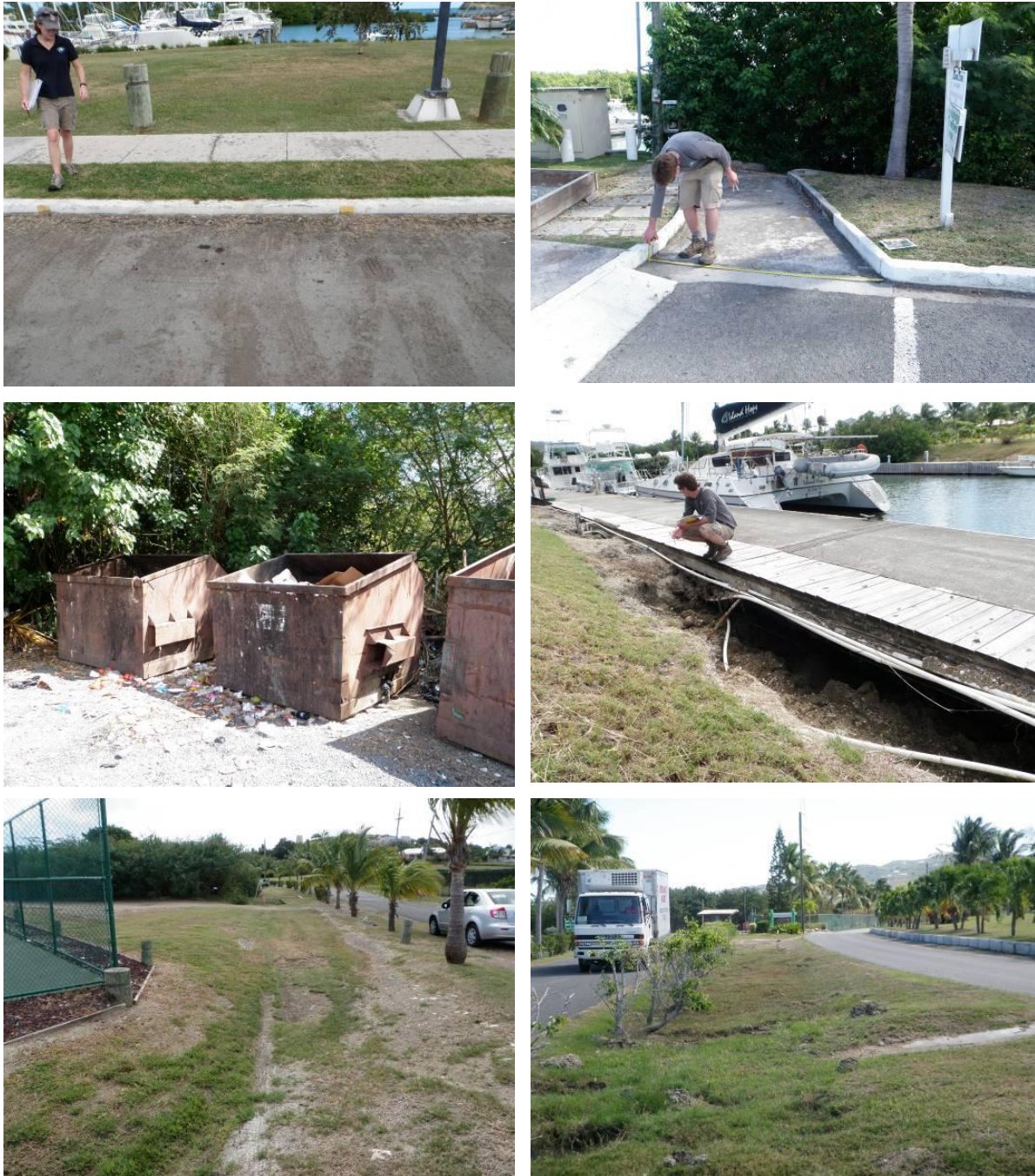
Figure 3.13. (Top left to right) Areas for bioretention and oil grit separator, (middle left to right) dumpster management and bulkhead stabilization, and (bottom left to right) areas for road drainage improvements (SG-R4-5).
