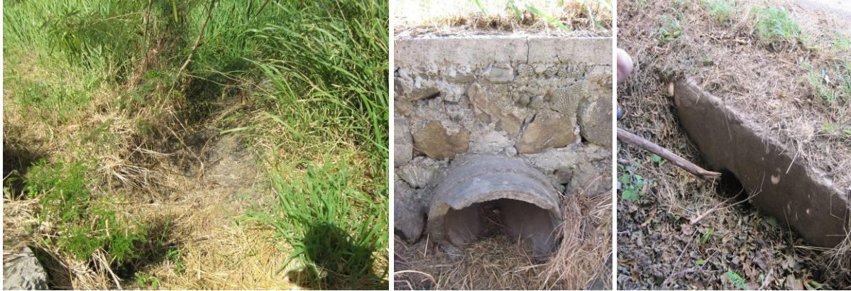
Figure 4.33. Erosion downstream from the first culvert (left); the second, chipped culvert (middle); and the partially blocked third culvert (right).
