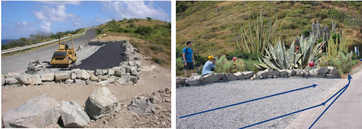
Figure 6.2. Construction of small parking lot at East End Bay Trailhead (left). Rendering of xeriscaped bioretention facility adjacent to parking lot (right).
