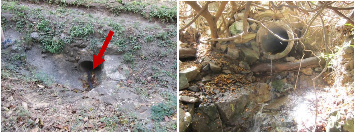
Figure 4.18. Arrow indicates PVC pipe discharging dry weather flow into culvert (left). Dry weather flow observed at downstream end (right).
