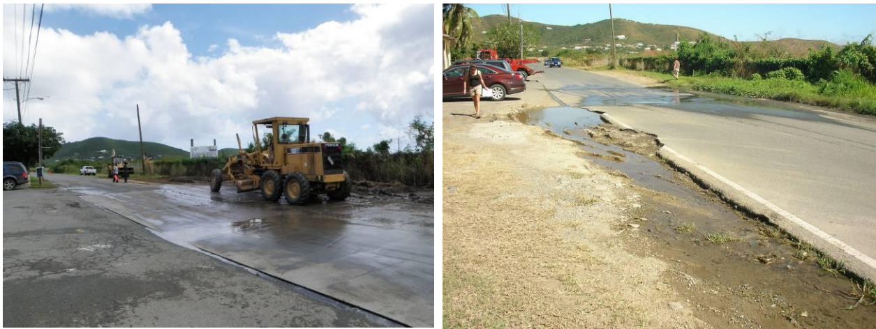
Figure 8.5. Road drainage issue in front of Milgie's Grocery.
