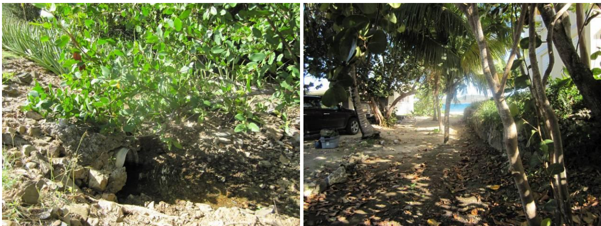
Figure 4.31. The second culvert underneath a driveway (left) leads to a shallow channel out to Yellowcliff Bay (right).
