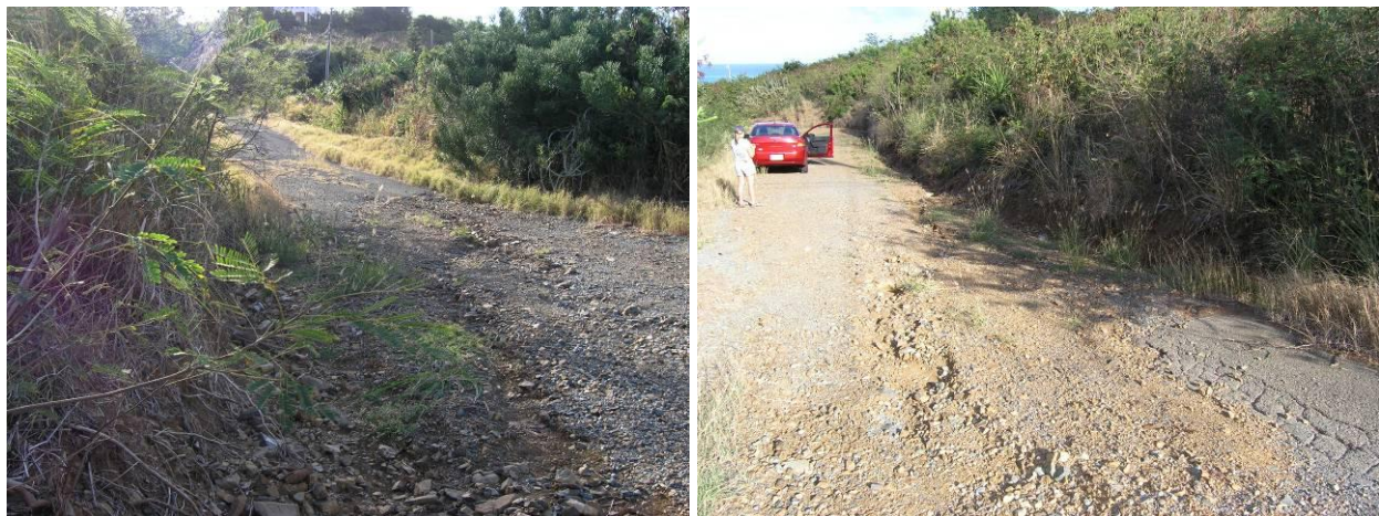
Figure 4.3. Erosion gully at the transition from paved driveway to unpaved private road looking up-gradient (left) and down-gradient (right).
