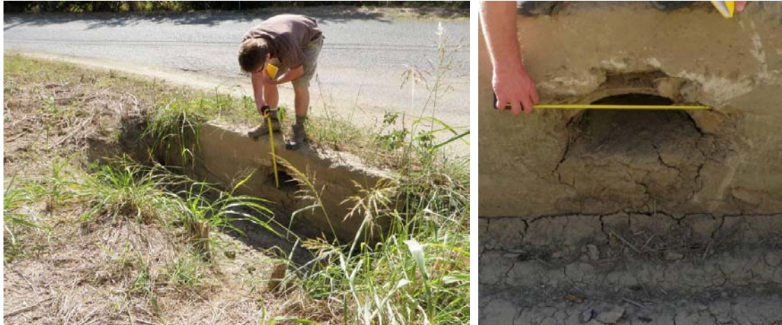
Figure 8.3. Unnamed road draining to South Shore Rd. deposits sediment across street into vegetated area and is contributing to road surface degradation.
