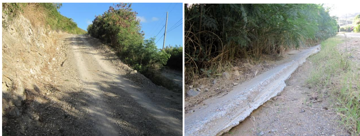
Figure 4.4. Roads in the Hope and Carton Neighborhood are unpaved and very steep (left). Runoff from this road bypasses and undermines the paved swale (right).
