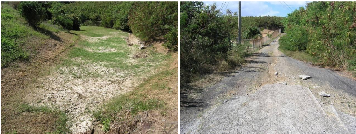
Figure 4.29. A pond is located upstream from the culverts – dry at the time of observation (left). The road itself is deteriorating and providing a sediment load to the gut (right).
