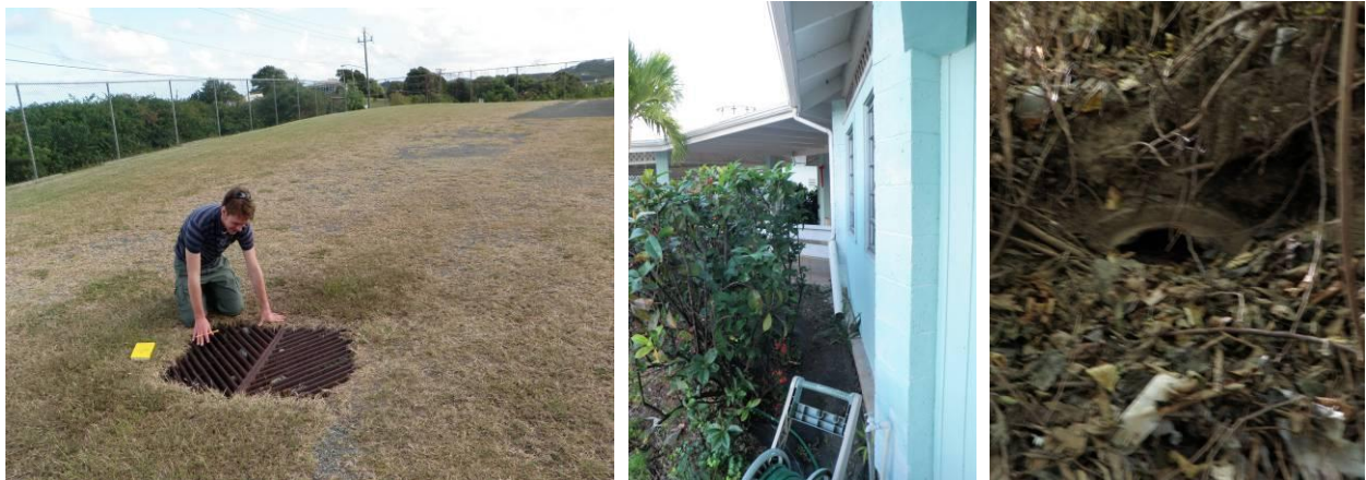
Figure 3.12. Drain inlet in lower parking lot (left); downspout to existing flowerbed that could be converted to a rain garden or collected for irrigation (middle); almost completely blocked culvert (right).
