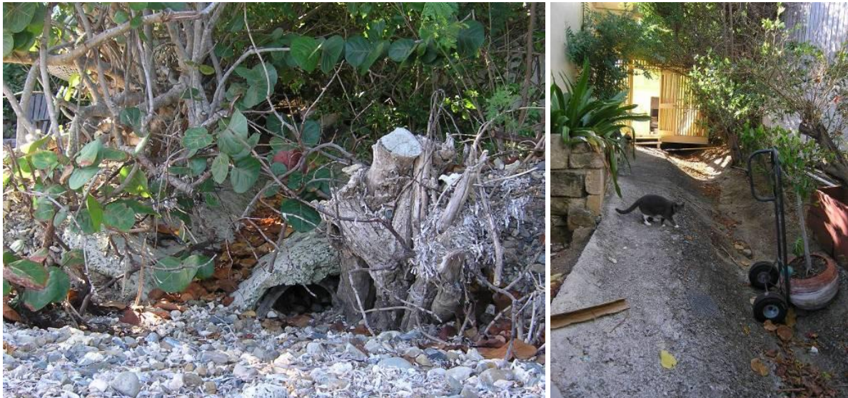
Figure 4.13. The outlet of the culvert is barely visible from the beach, with a crumbling concrete swale on top of it (left). Better view of the concrete swale constructed to convey runoff that overflows over East End Rd. between two private residences, bypassing the culvert (right).
