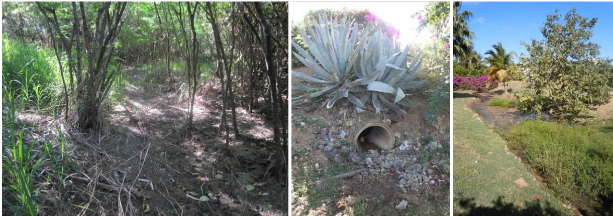
Figure 4.30. The gut upstream from the culvert (left). The downstream end of the culvert (middle). Ponded water in the front of a private residence (right).
