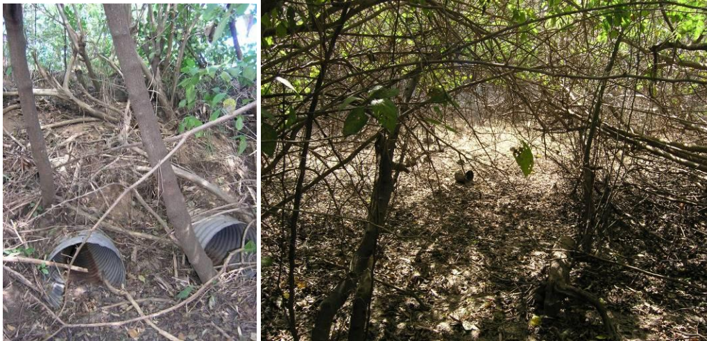
Figure 4.24. Two 24-inch CMP culverts that cross an unnamed road (left). A depression exists at the upstream end that only holds water in the wet season (right).
