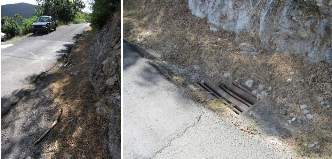
Figure 4.35. Blocked inlet to this culvert on Seven Flags Rd.
