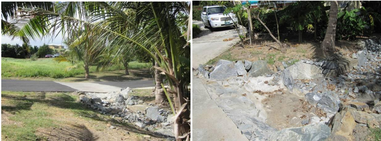
Figure 4.21. Stormwater flows from the grass depression and the cul-de-sac to a riprap-lined channel (left). A sediment forebay was constructed with a rock weir (right).
