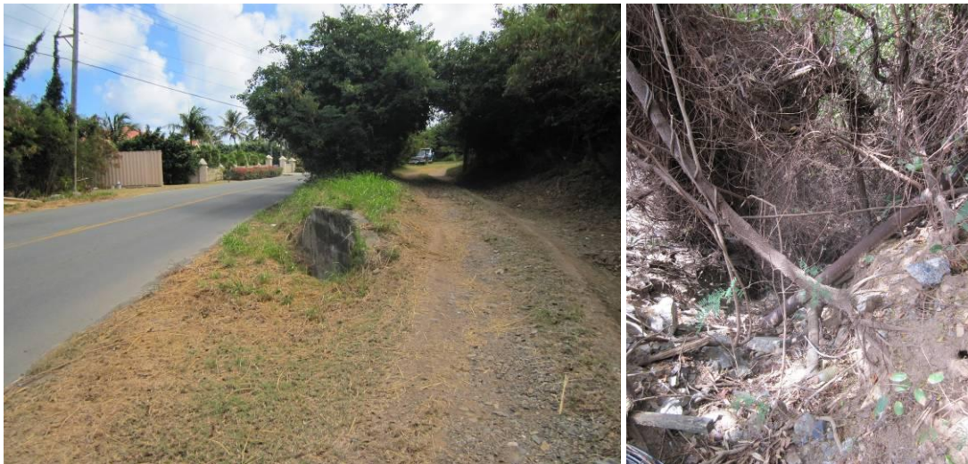
Figure 4.34. Upstream end of culvert has large headwall separating it from an unpaved drive (left); the downstream end is scoured out and clogged with vegetation (right).
