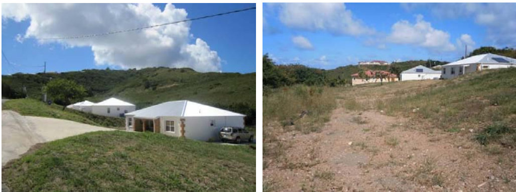
Figure 4.7. New homes were built in the gut upstream from the Seven Flags Rd. erosion (left). The areas behind the houses should be retrofitted to create a series of terraced depressions to help provide more storage and decrease velocities (right).
