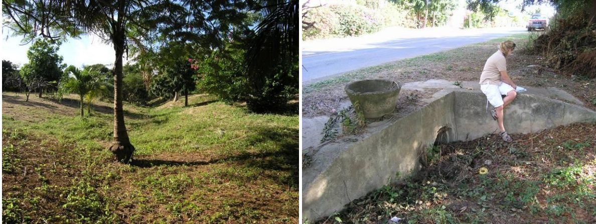
Figure 4.12. View upstream along one fork of the gut system (left). Concrete headwall for 15-inch reinforced concrete culvert (right).
