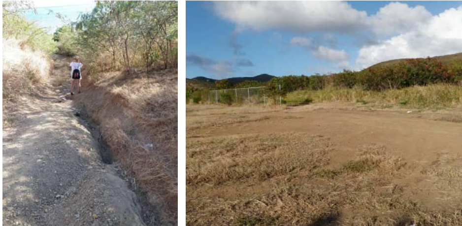
Figure 8.11. Eroded trail to beach (left) and parking area (right)
