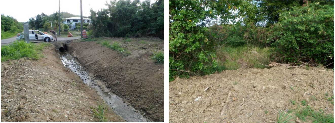
Figure 3.6. Missed opportunity to demonstrate water quality designs and proper soil stabilization techniques at newly installed culverts.
