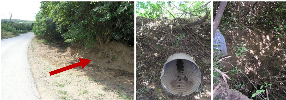
Figure 4.25. The arrow shows the sediment that gets cleared off Pony Club Trail and pushed into the gut (left). The upstream end of the culvert is clear of debris and is in generally good shape (middle); however, a large scour hole has formed at the downstream end (right).
