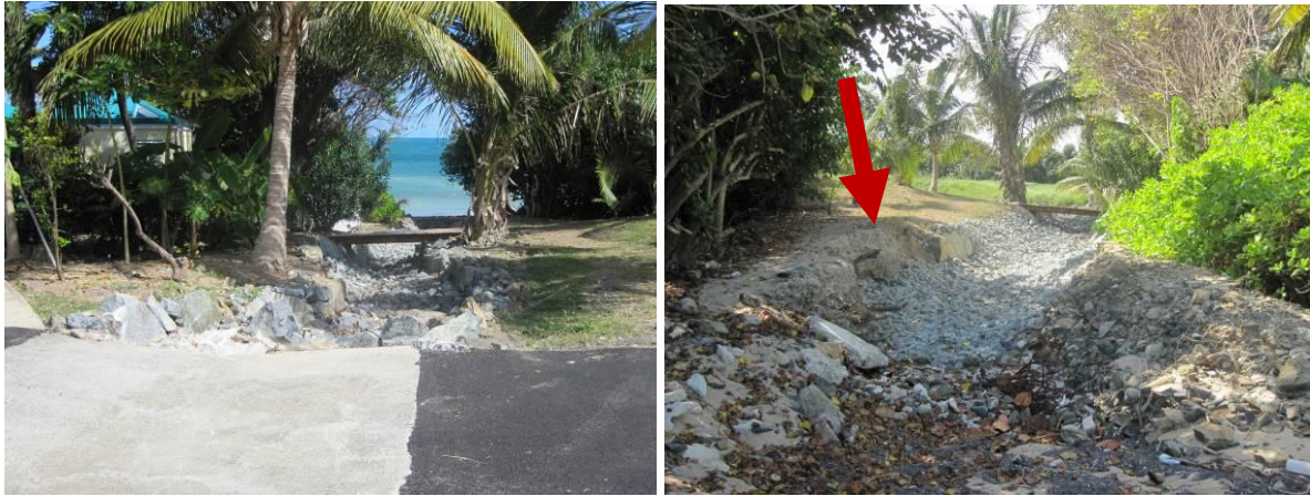
Figure 4.22. The channel flows directly to Coakley Bay (left). A portion of the downstream end of the channel has eroded (right).
