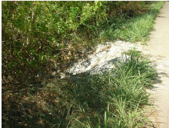
Figure 8.8. Attempt at concrete flume to manage runoff on East Maria Lane above culvert (GP-RC-4).
