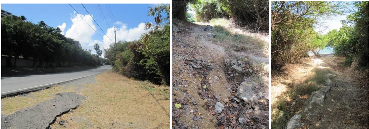
Figure 4.19. Runoff from Coakley Bay Condos flows across East End Rd. and down a beach access road (left) causing erosion gullies (middle), and this sediment-laden runoff enters Coakley Bay (right).
