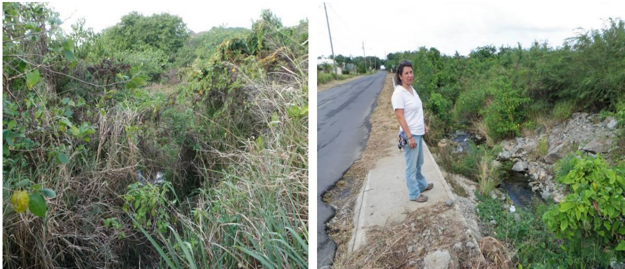
Figure 3.8. Well vegetated banks of west gut on Schuster's property (left) and example of on-going road repair and bank stabilization efforts along South Shore Rd. (right).
