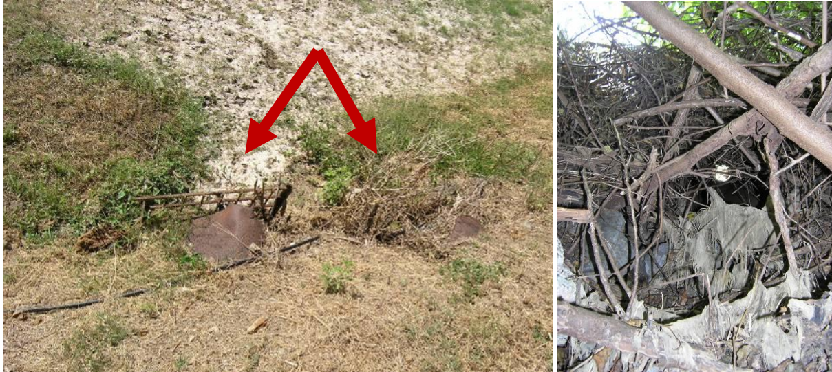
Figure 4.28. The two 24-inch ductile iron culverts have damaged trash racks – one made of rebar grate and one made of wire fencing and sticks (left). The downstream end is clogged with vegetation (right).
