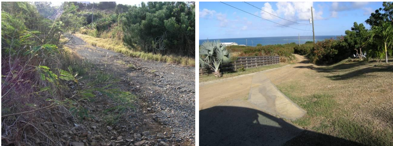
Figure 4.37. Erosion along private road within Sierra Verde neighborhood at meeting point between paved and gravel roadways (left) and water bar installed along main dirt road in Sierra Verde neighborhood.
