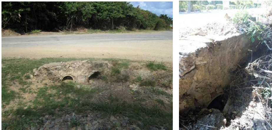
Figure 4.6. The two culverts that carry flow from Seven Flags Rd. and a portion of East End Rd. to Solitude Bay blocked with sediment on both the upstream (left) and downstream ends (right).
