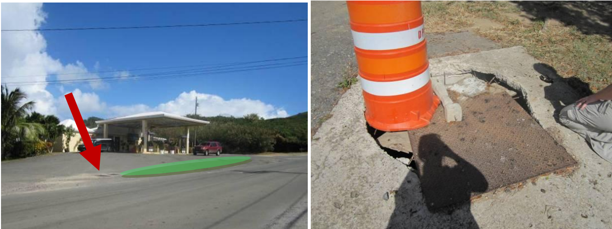
Figure 4.15. Some pavement could be removed at the gas station to create a treatment swale (shown in green) up-gradient from the existing catch basin indicated with an arrow (left). Manhole covers are missing all along the 48-inch culvert leading out to Coaklely Bay, creating a safety hazard (right).
