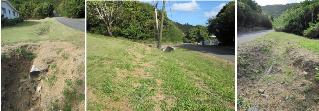
Figure 4.32. Erosion caused by deteriorating culverts in the southern portion of Pleasant Valley.
