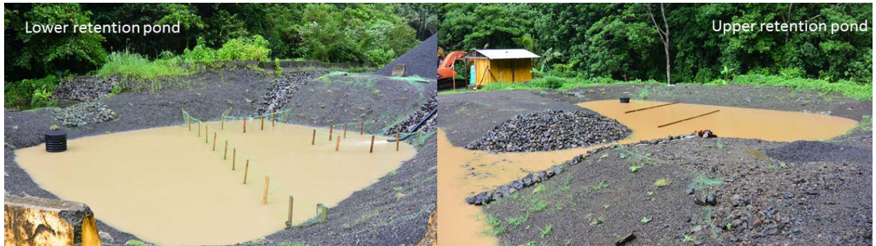
Figure 7. Pictures of the Lower and Upper retention ponds at the Samoa Maritime Quarry, full of sediment-rich runoff following a large rain storm. Both were installed in September-December 2014. The Upper retention pond (right) is a two-pond configuration, connected by a rubble-lined spillway. Stand-pipes are visible in the corner of each retention pond. During major rain events these route water from the pond directly into the stream to prevent overtopping the retention pond banks. Pictures taken by Alex Messina.
