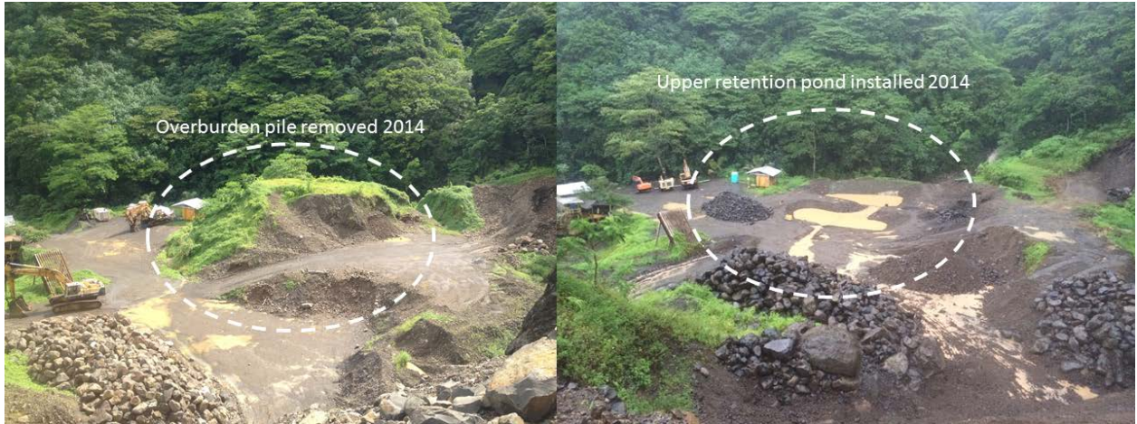
Figure 6. Pictures of the Upper Operational Area/Excavation Platform before (left) and after the installation of the Upper Retention Pond. A similar retention pond is also installed at the Lower Operational Area (not shown).
